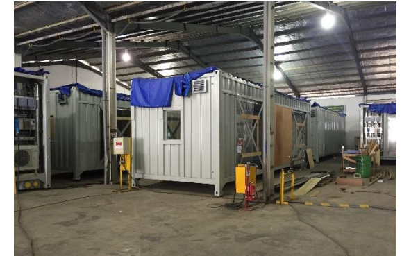
Hebron TLQ – BP Fabrication of module sections at Profab Yard, Batam, Indonesia – 2015
