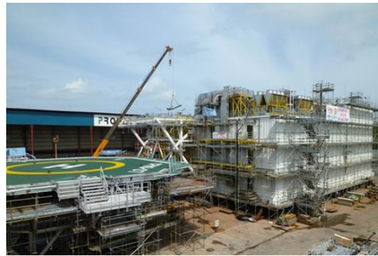
Champion 7 – Brunei Shell Petroleum Module Fabrication in Emtunga's workshop in Emtunga, Sweden and final assembly at Profab Yard, Batam, Indonesia – 2012
